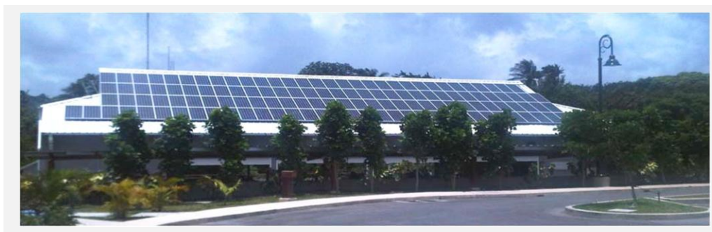
Figure 1.6. Use of photovoltaic technology to generate electricity at the redeveloped Harrison's Cave in St. Thomas.
