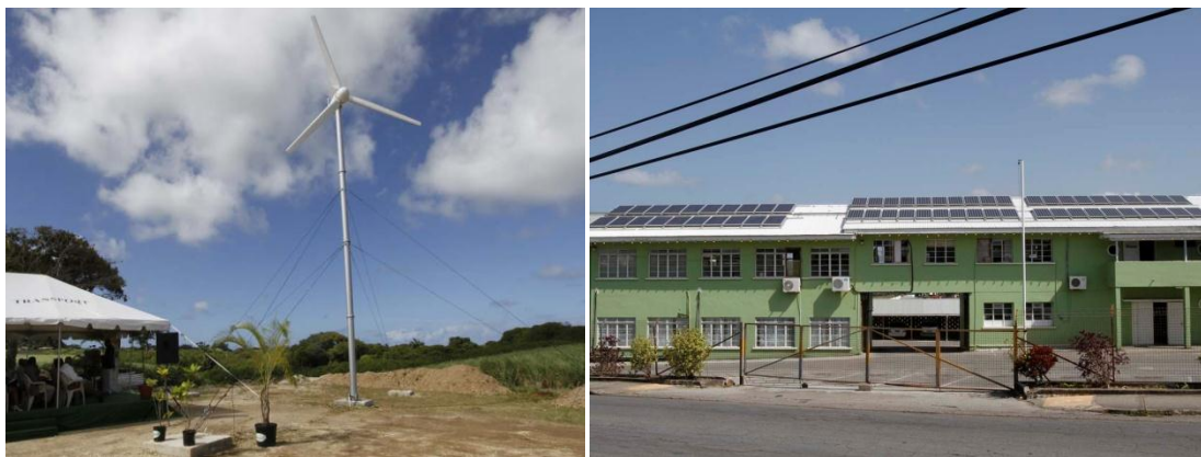
Figure 1.7. Examples of renewable energy installations in Barbados: Wind turbine in St. Lucy (left); photovoltaic panels on the Ministry of Public Works’ office building (right).
